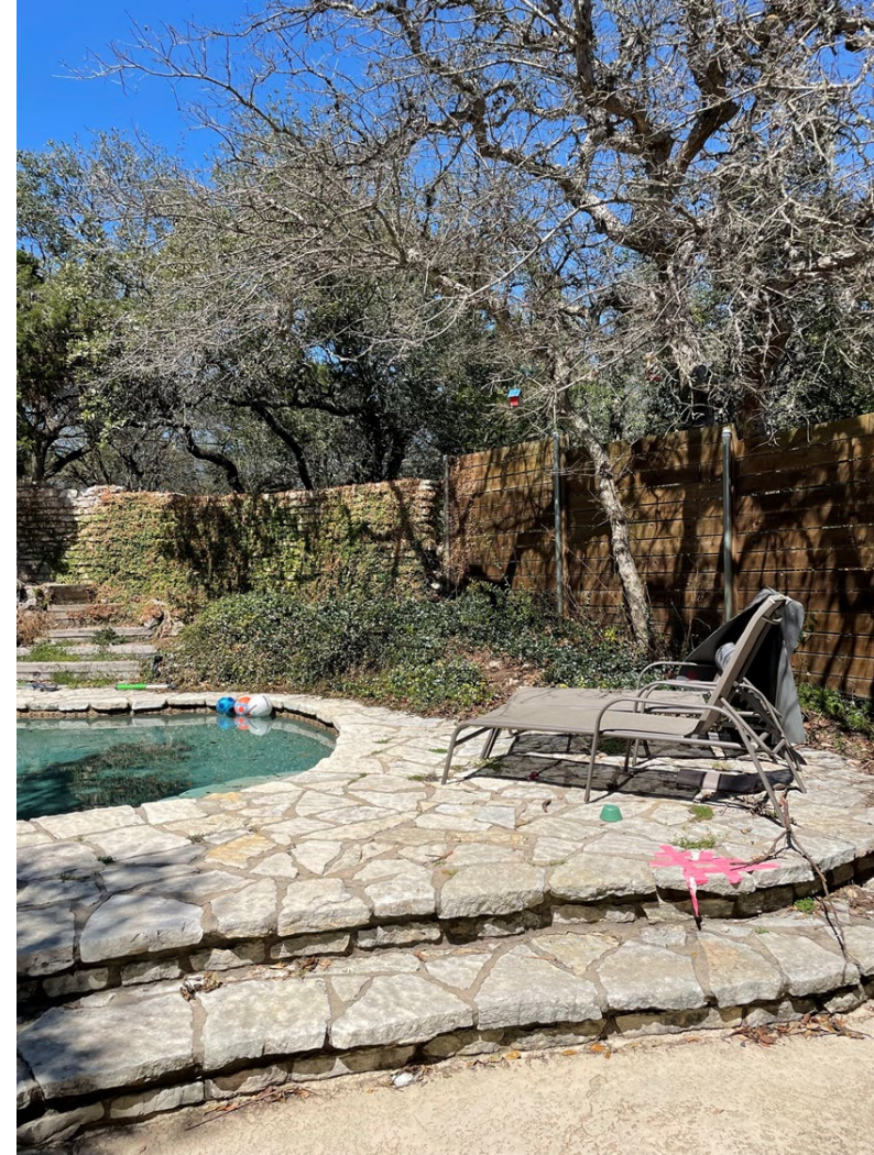
VIEW 6 – POOL DECKING TO BE REPLACED THIS AREA, 6" DIA. OAK TO BE REMOVED AND REPLACED, WOOD FENCE TO BE REMOVED
