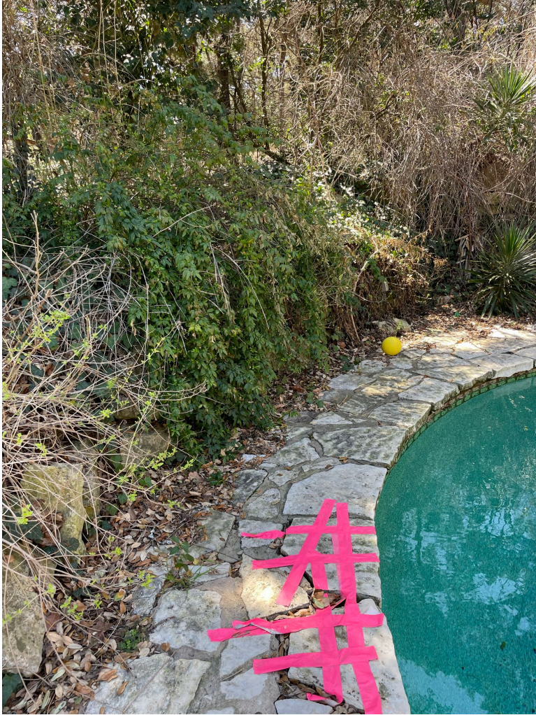
VIEW 13 – STONE POOL DECK AND COPING TO BE REPLACED
