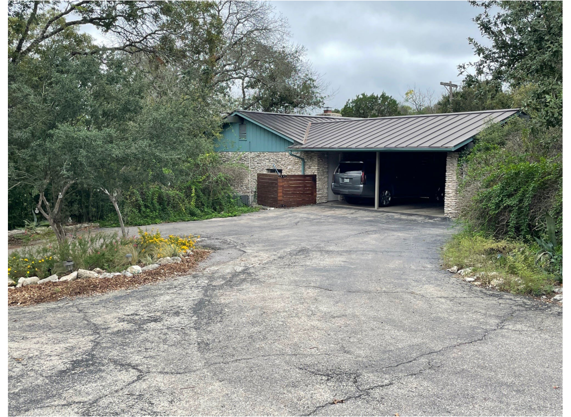
VIEW 2 – DRIVEWAY ENTRANCE VIEW TO CARPORT - PAVING TO BE REPLACED
