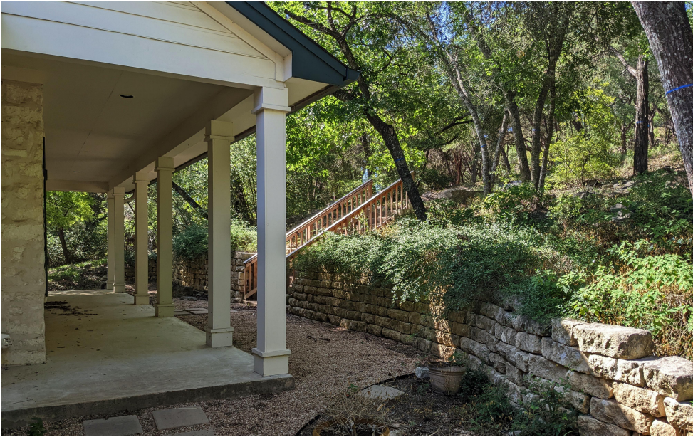
EXISTING (NON-COMPLIANT) CUT AREA
