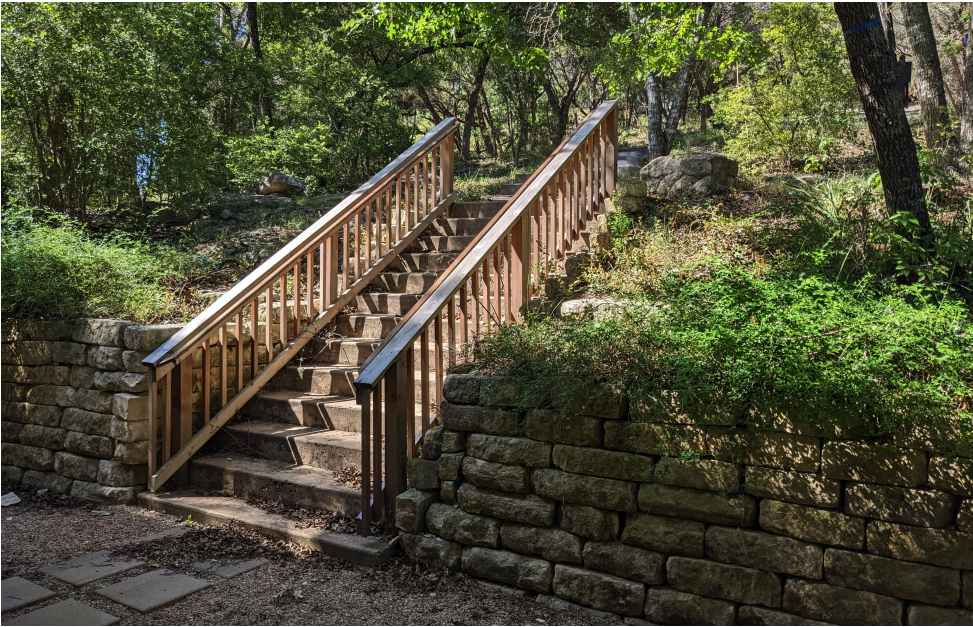
EXISTING (NON-COMPLIANT) SITE WALL
