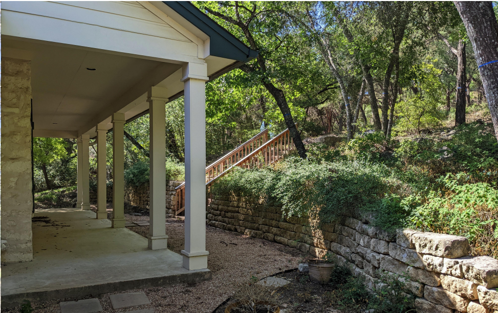
EXISTING (NON-COMPLIANT) CUT AREA
