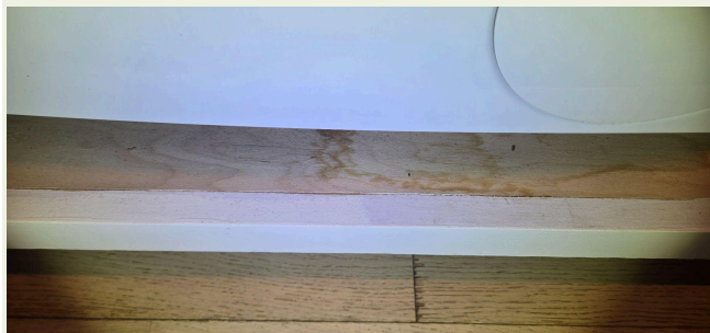
Evidence of prior water leak.
