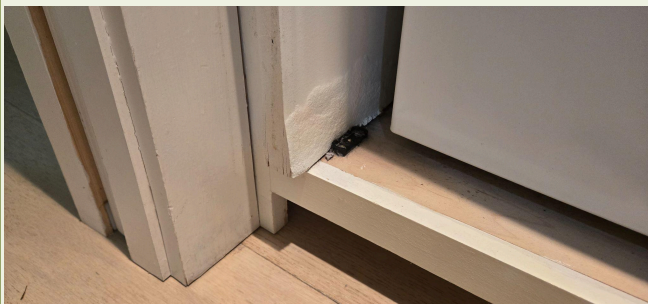
Evidence of past water damage to the cabinet gable.
