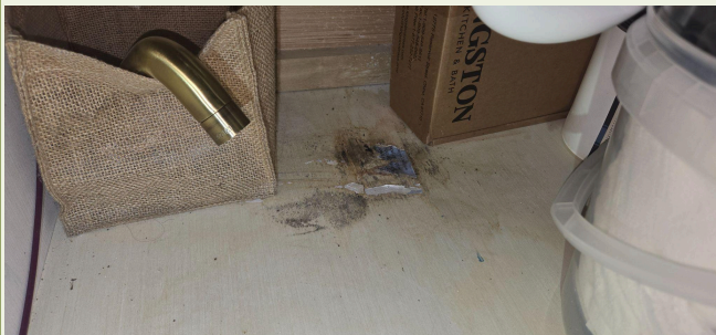
Likely mold accumulation from plumbing leak.
