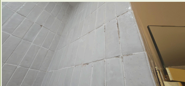
Deteriorated shower grout
