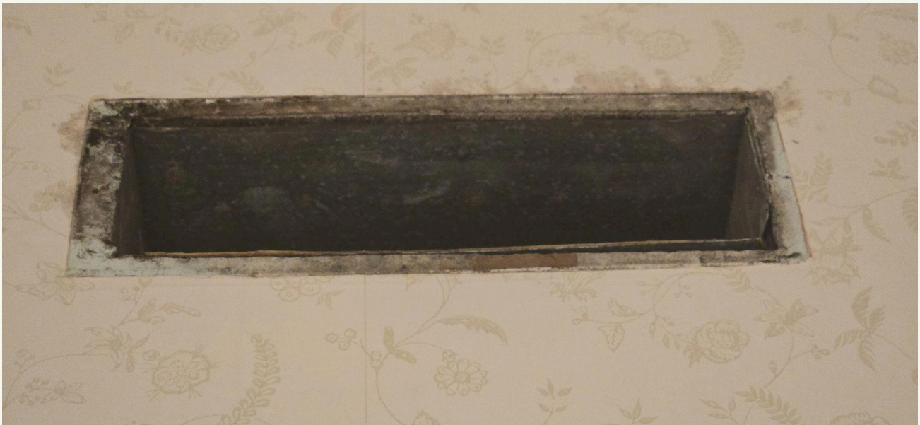
Photo #02 :CRITICAL: Mold growth detected around supply air boot, drywall and wallpaper in daughter's bedroom.
