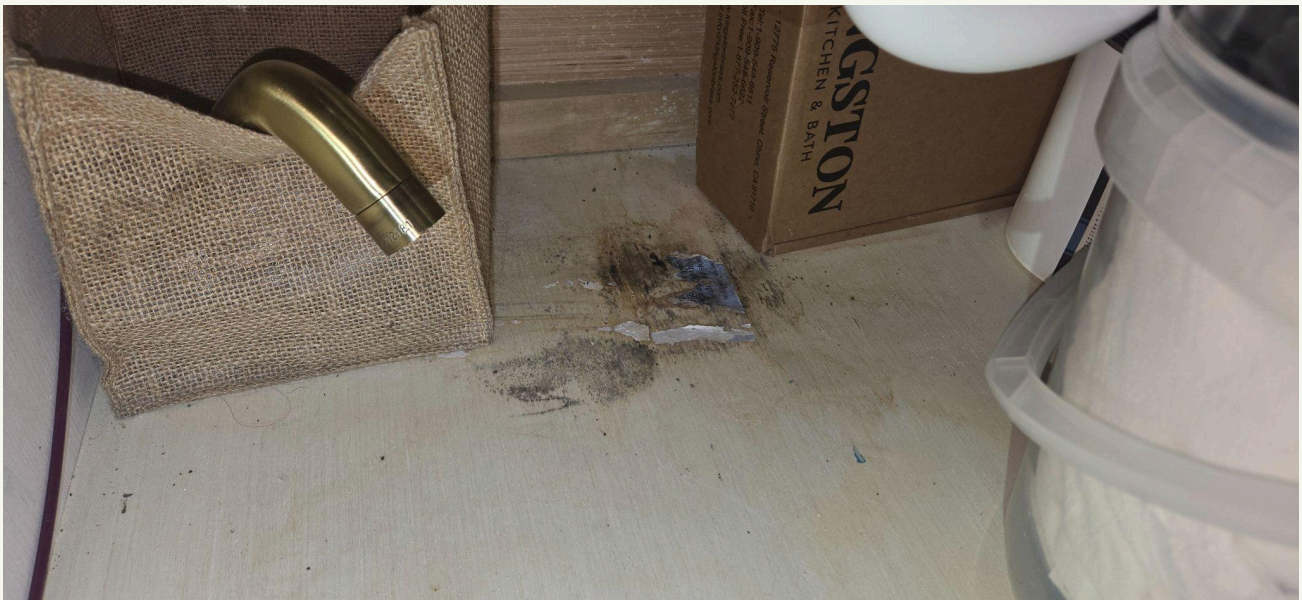
Photo #03: SIGNIFICANT: Suspected mold growth observed in guest bathroom vanity likely due to prolonged water dripping from loose plumbing fitting.
