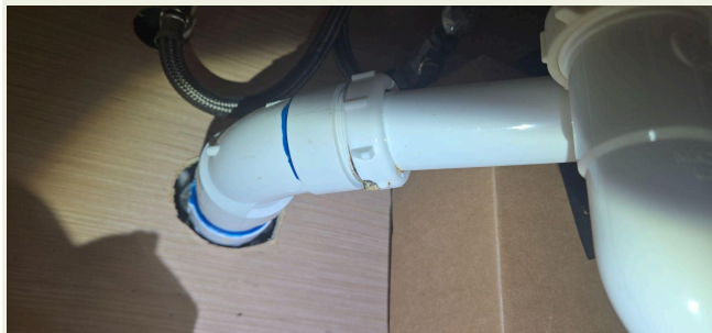
Evidence of slow leak from plumbing line above staining
