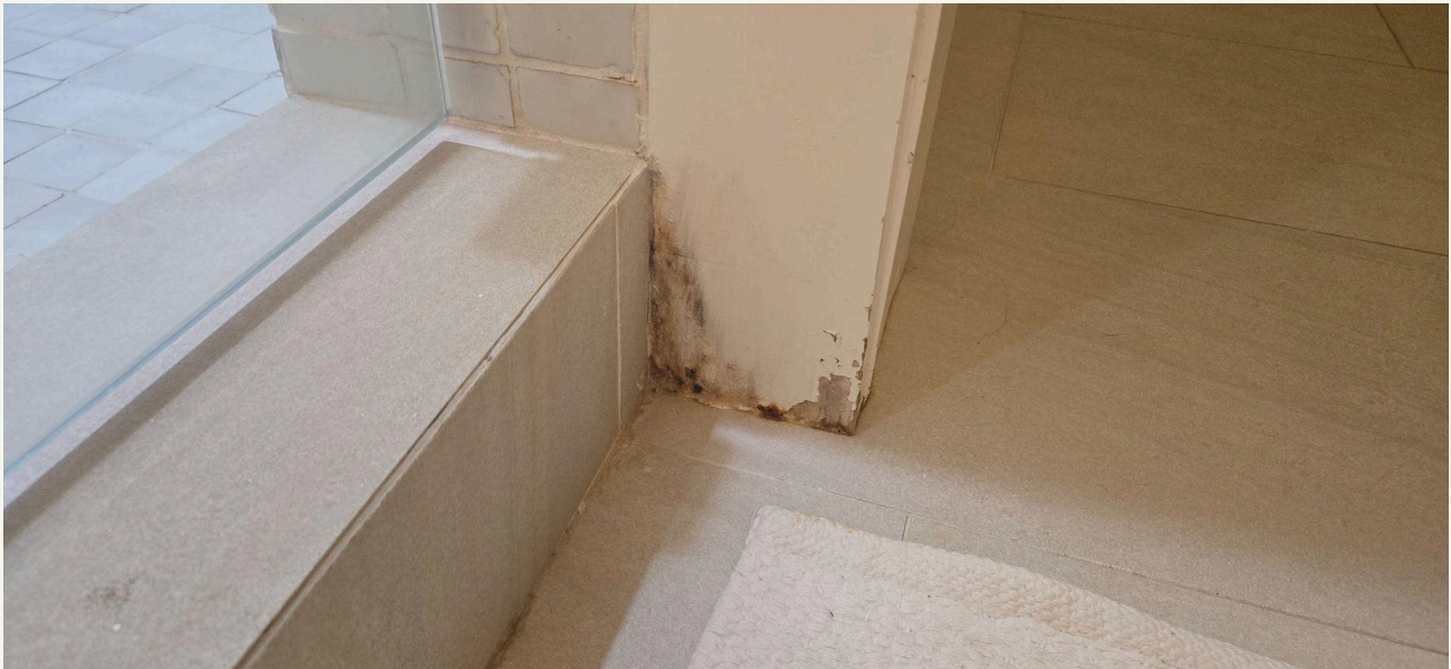
Photo #01: CRITICAL: Active mold growth adjacent to shower.
