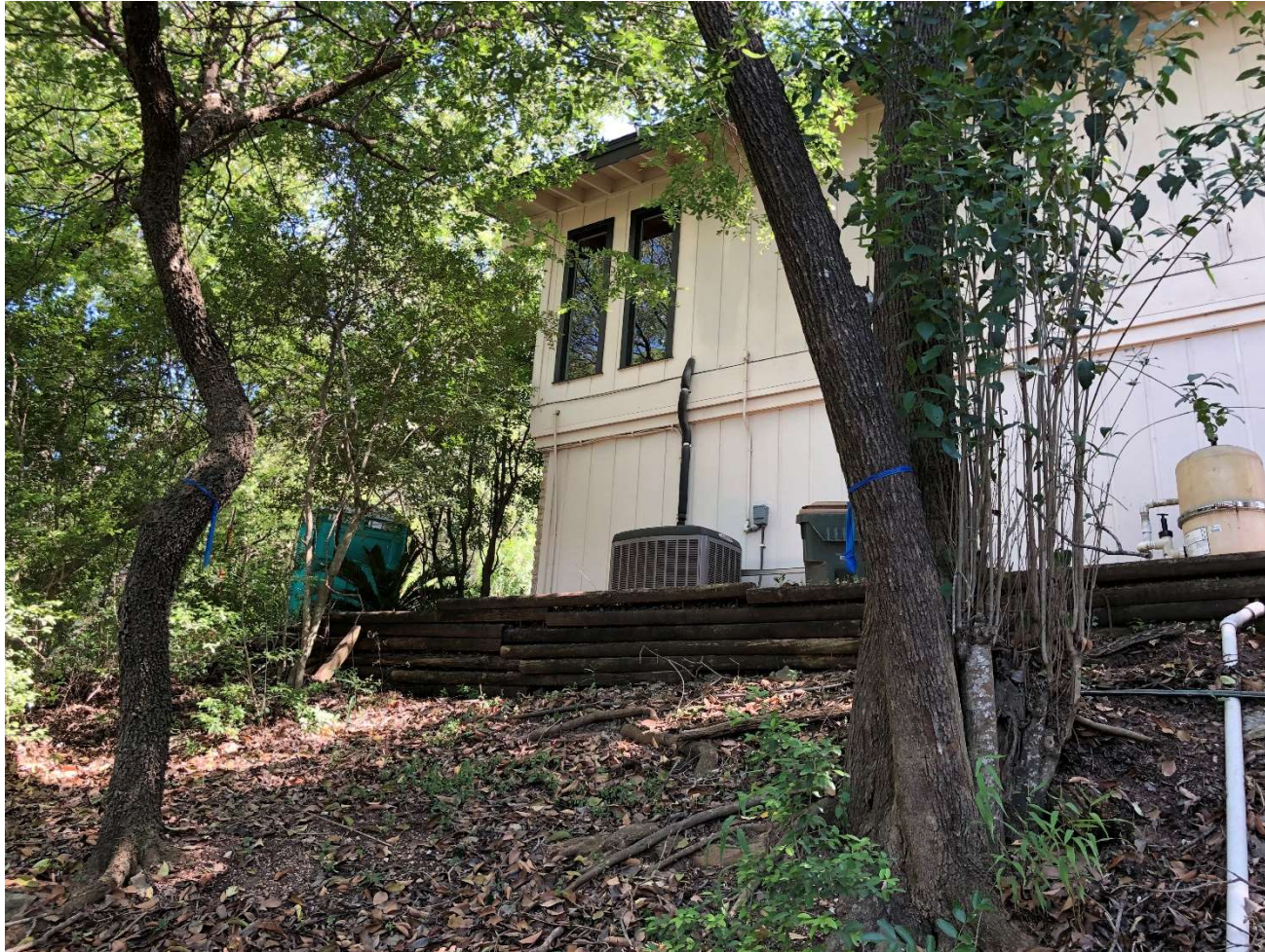
This is a view on the right side of the house, showing the old woodend retaining wall that is failing. The wood timbers are separating and bulding out.
