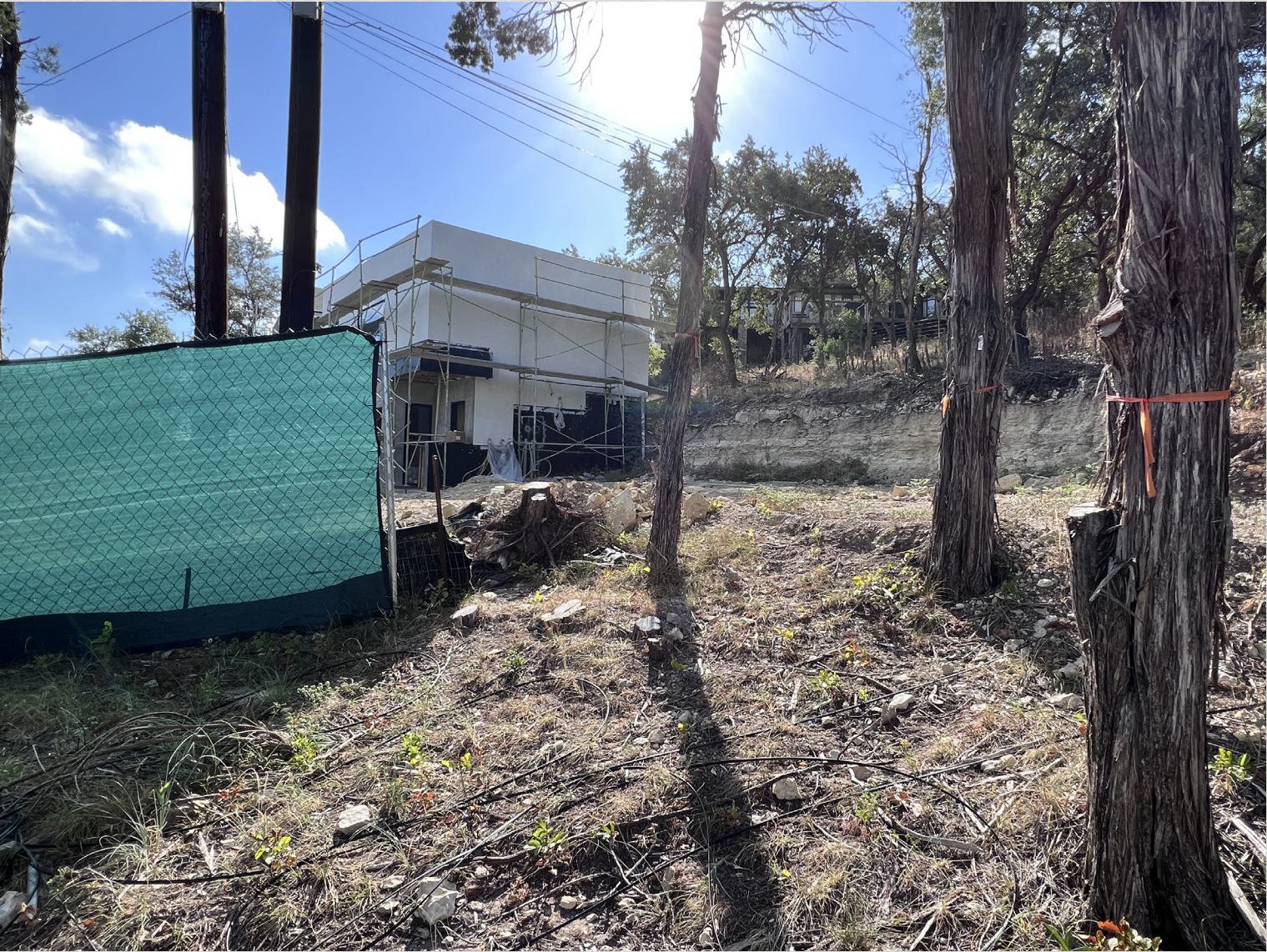
Home Across the Street Appears Extremely Tall with Large Grade Cuts & Retainage
