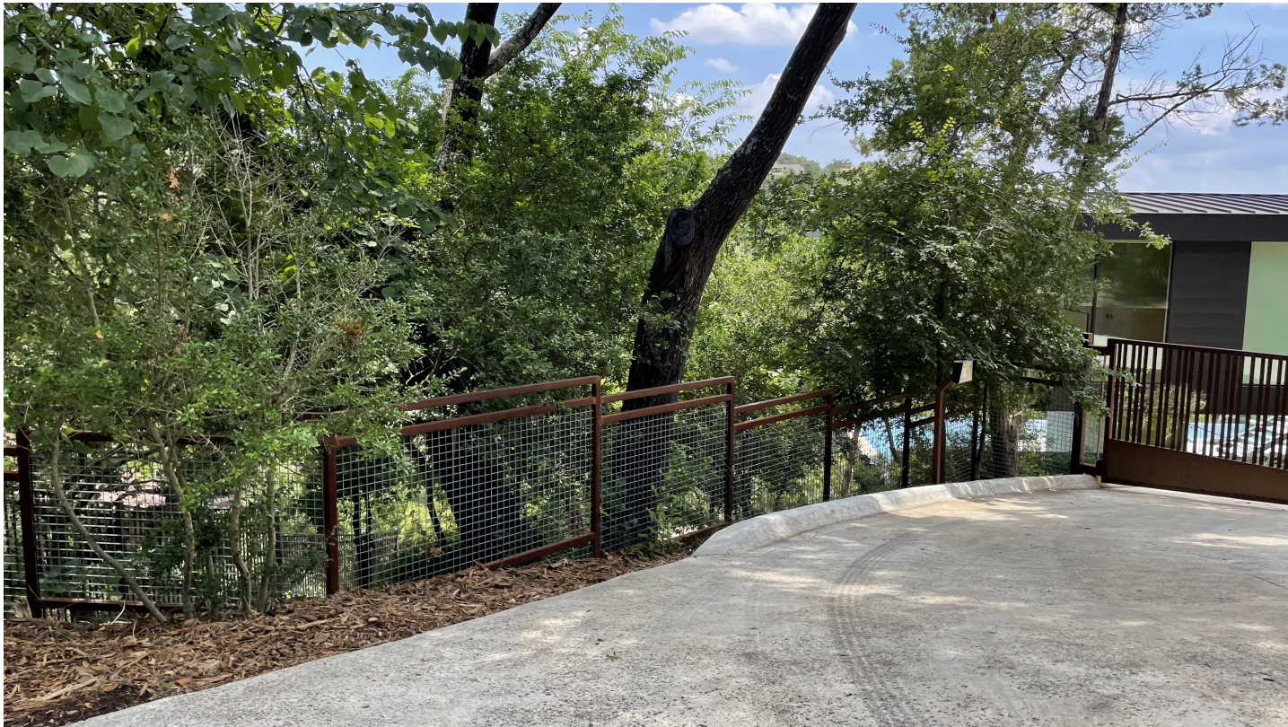
1. PERIMETER STEEL FENCING WITH WELDED WIRE MESH PANEL
